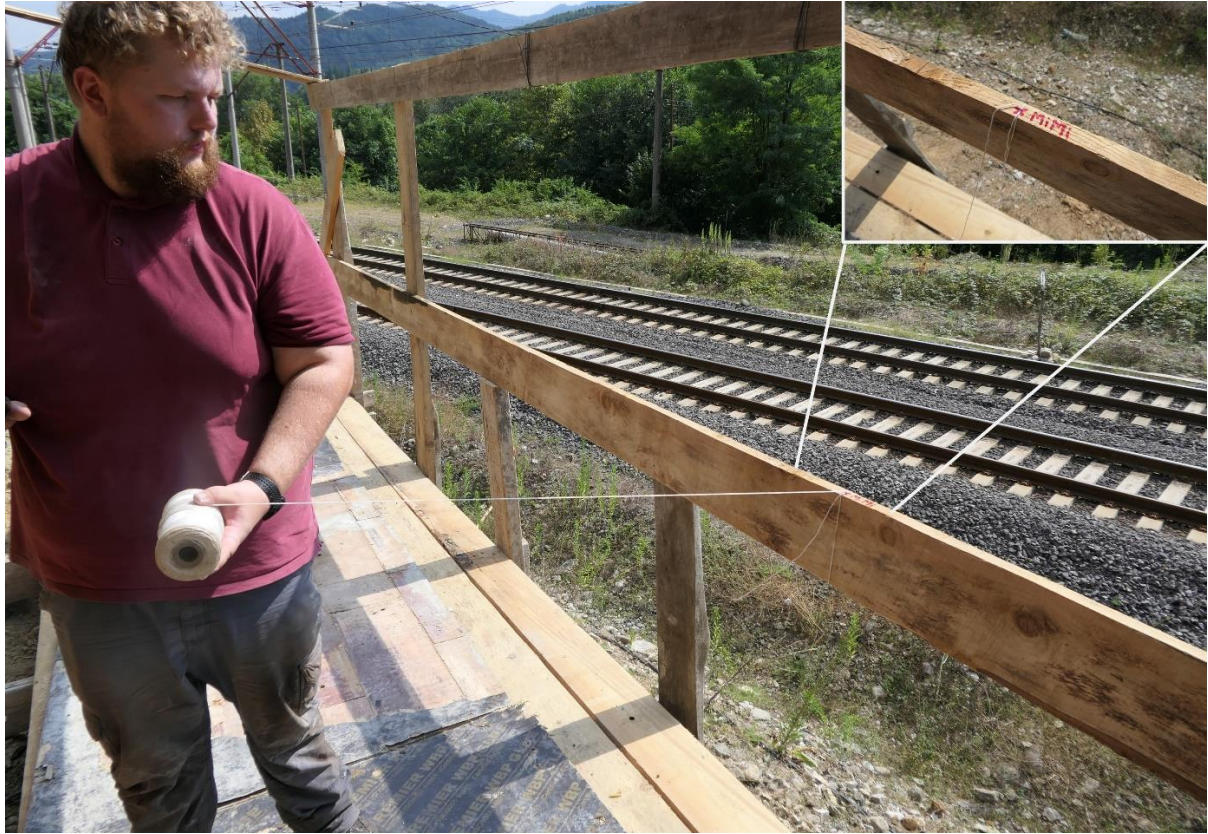
Figure. 3. We took the elevation of the block samples from the illustrated point in the excavation balcony.
